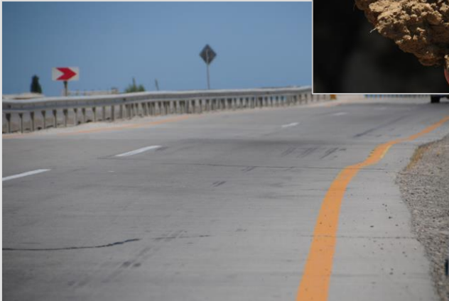
Deformed slabs resting on settling foundations
